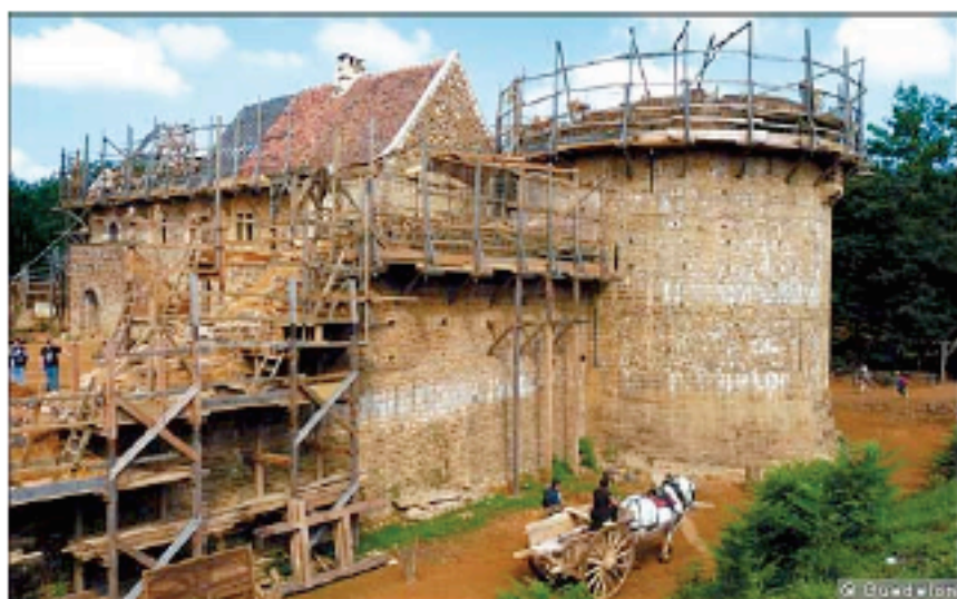
A team of 40 workers is building a replica of a 13th-century castle in the forest of Guddelon in Burgundy without using power tools, in a project that is being financed by paid visitors
